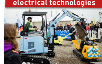
Demonstration building site electrical technologies
